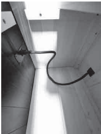
Heater Power Cable
