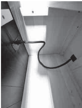
Heater Power Cable
