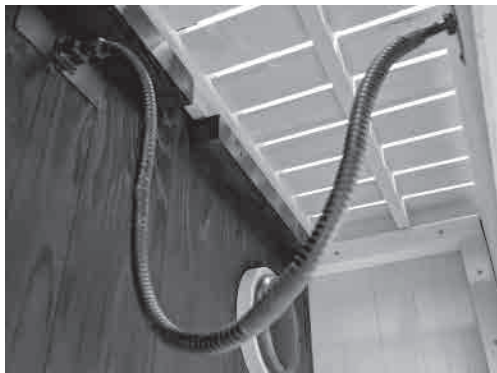
Heater Power Cable
